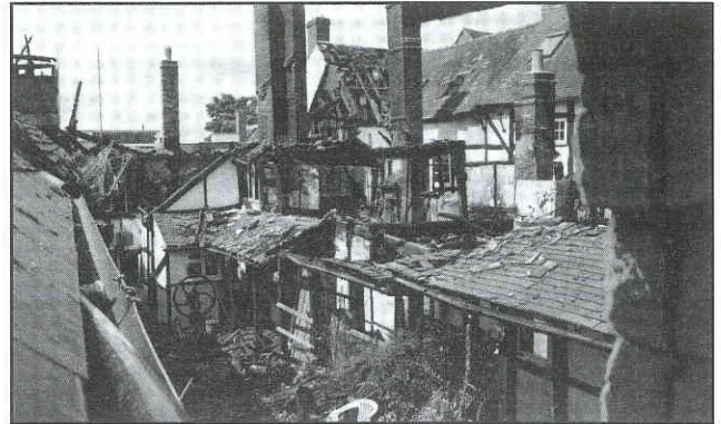
Fire damage at the rear of the Seven Stars
