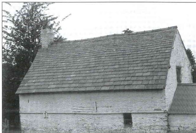
The reroofed Lower Llanon Farmhouse, Urishay with stone slabs from the Coed-Major Delve
