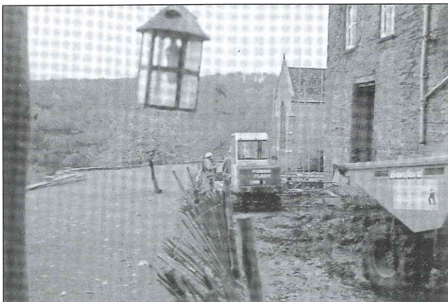
Work in progress on the eastern side of the Dinmore complex, with the medieval church beyond. The scaffolding lamp adds a curiously seasonal touch!
