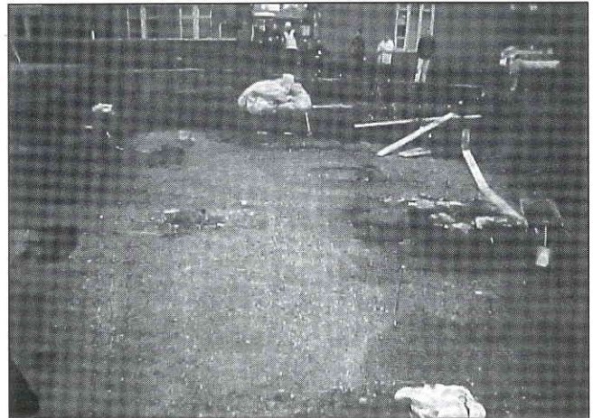
Excavations in progress at the site of the new Magistrates Court, Hereford.
